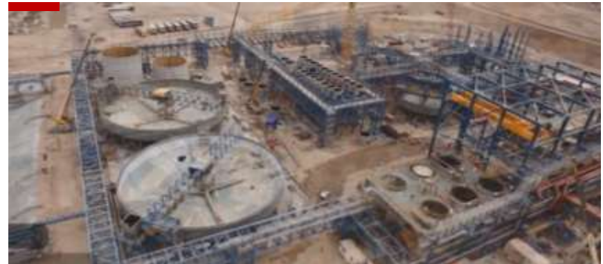
▪ Concentrate thickening, Molybdenum plant
