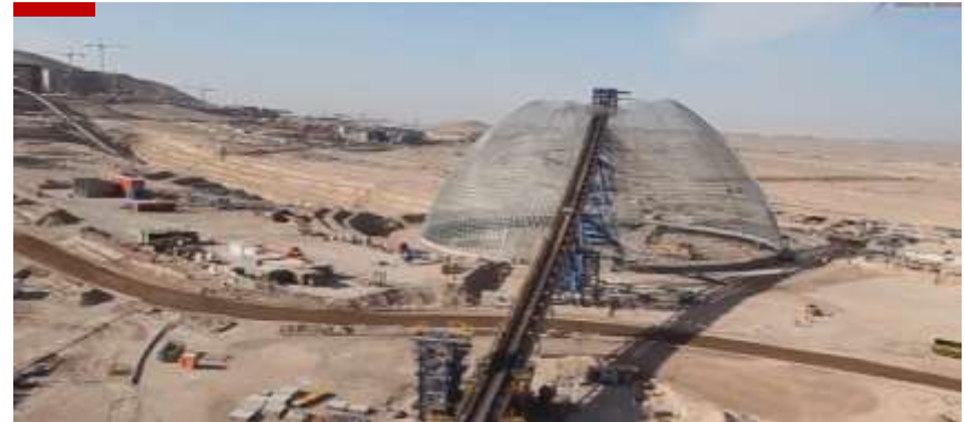
▪ Crushed ore storage facility
