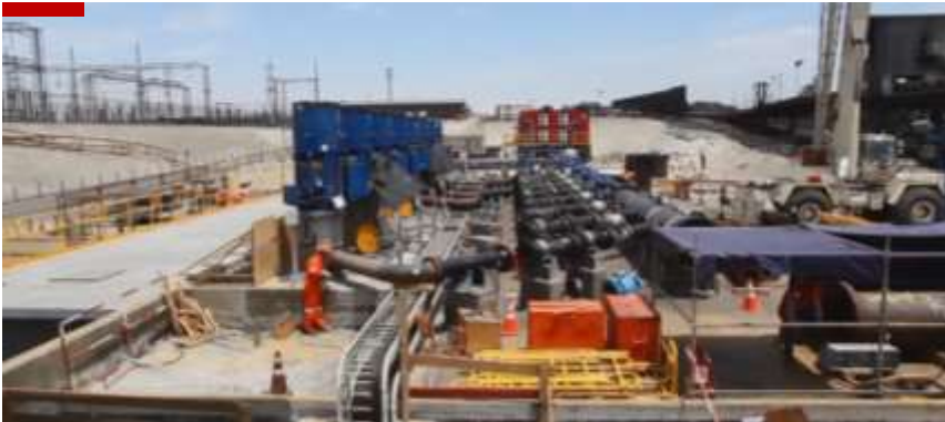
▪ Sea water pipeline – coastal station
