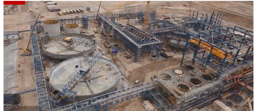
▪ Concentrate thickening, Molybdenum plant
