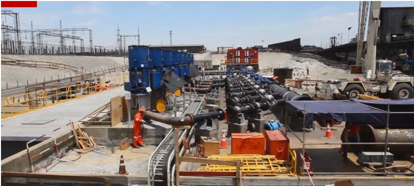
▪ Sea water pipeline – coastal station
