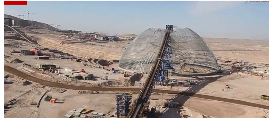
▪ Crushed ore storage facility
