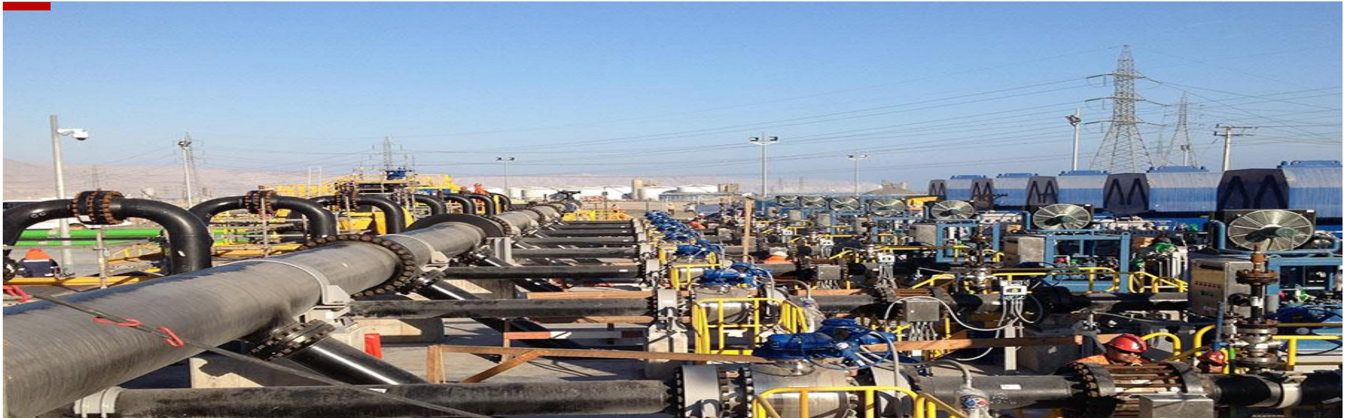
Sea water pipeline and pumping station
