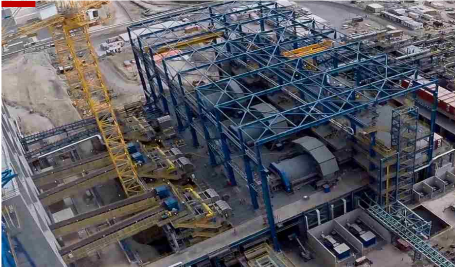
Ball mills (also visible: conveyor belts and tertiary crushers)
