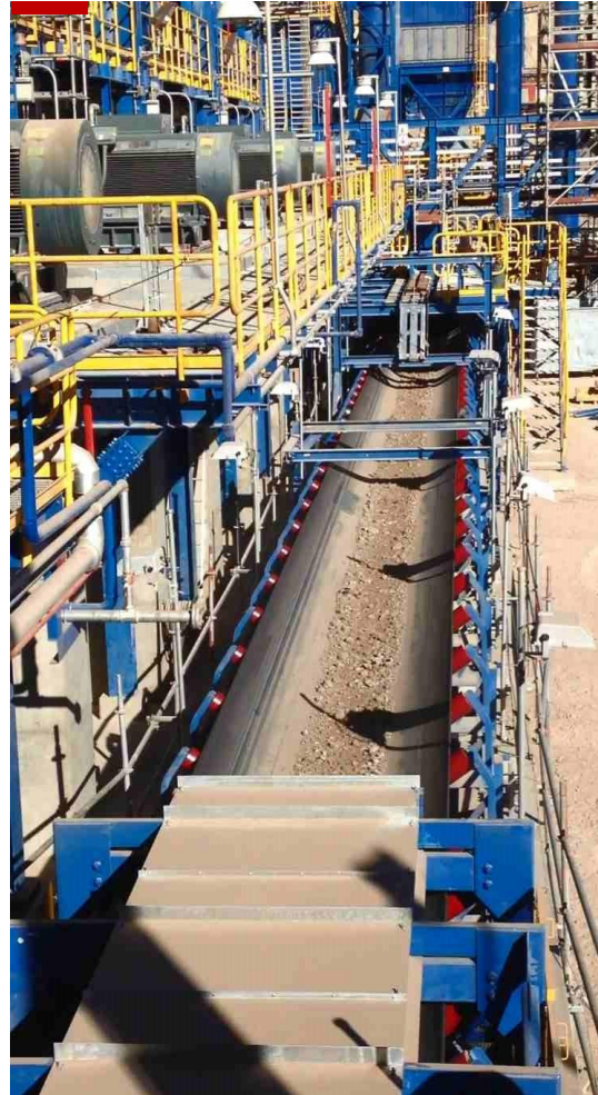
CV-160 conveyor belt with the first load of fully-crushed ore being transported to the fine ore bin
