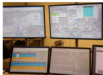
Main Control System
