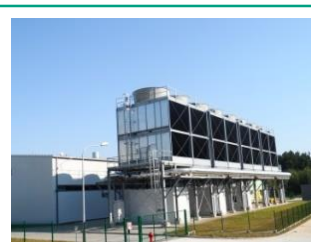
Cooling tower and heat transfer building
