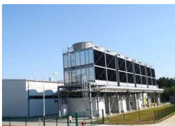
Cooling tower and heat transfer building
