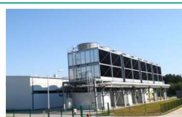
Cooling tower and heat transfer building
