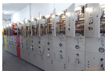
Main Control System
