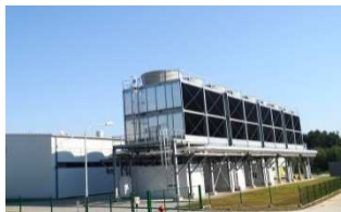
Cooling tower and heat transfer building
