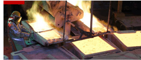
Construction of a second flash furnace and modernisation of the Głogów Smelter
