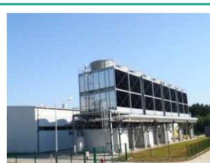
Cooling tower and heat transfer building
