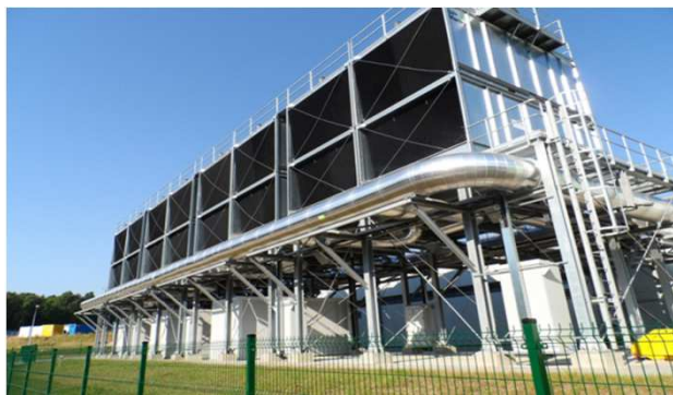
Cooling Station at R XI shaft – heat transfer tower
