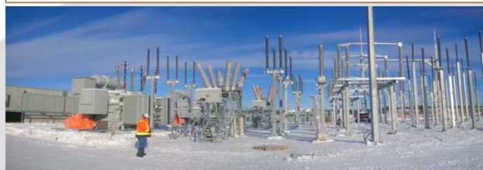
230 kV transformer station (Victoria)
