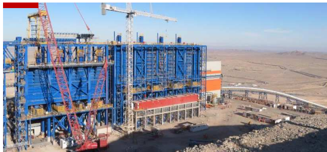
▪ Secondary Crusher & HPGR
