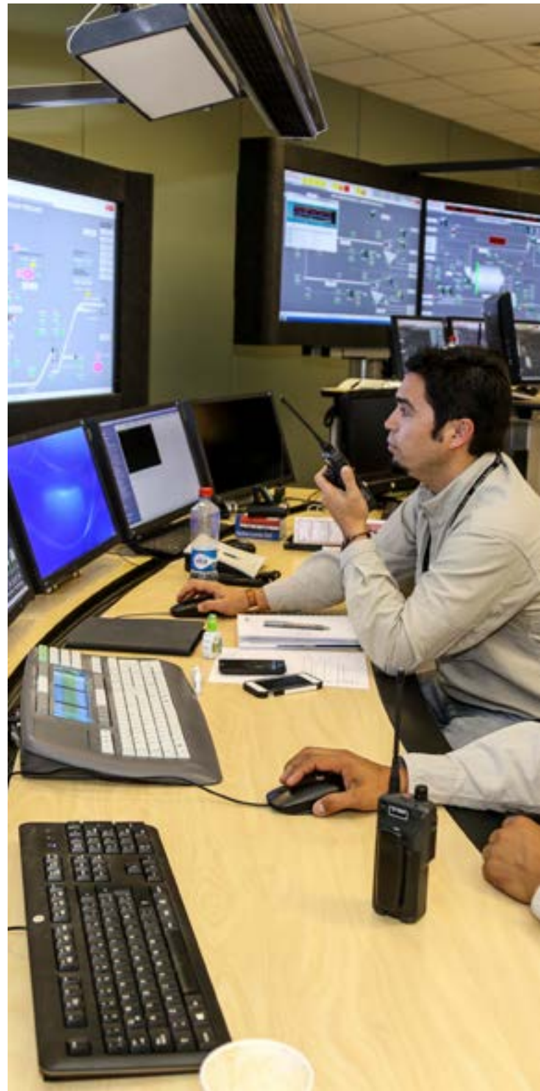
Control room - Sierra Gorda mine, Chile
