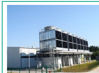
Cooling tower and heat transfer building
